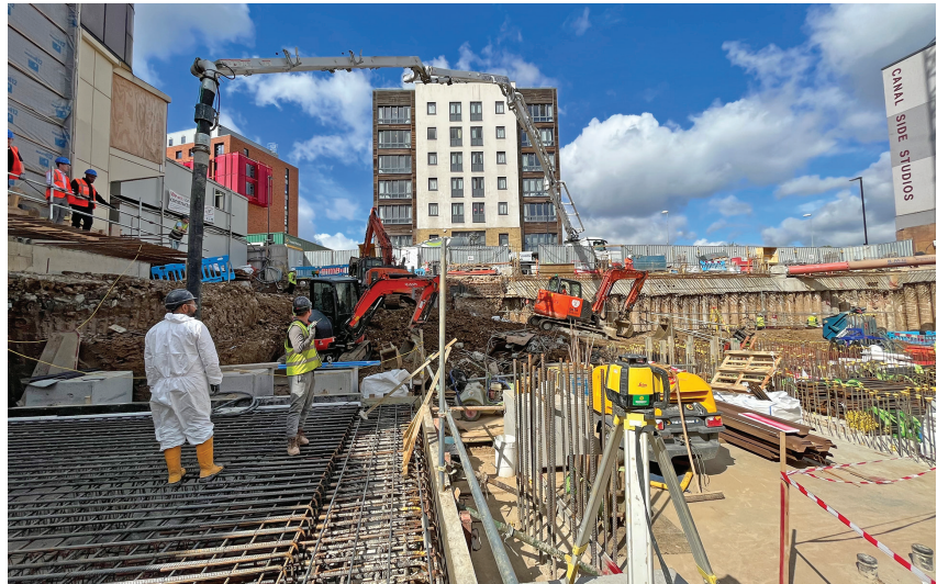
Pump pipe (rear centre) delivering MagnaDense concrete to cover the sewer (front left).
